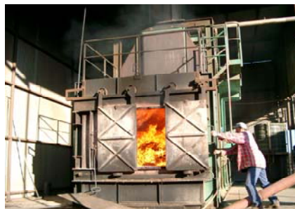
Spent charge fuelled steam boiler
